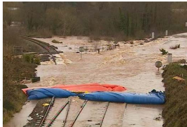
Flooding of the railway at Cowley, Exeter, UK – 20 Oct. 2014 (Photo from: https://www.networkrailmediacentre.co.uk/resources/ )
